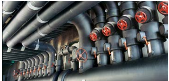
Many advantages described above making Aeroflex suitable for insulating chilled water piping.
